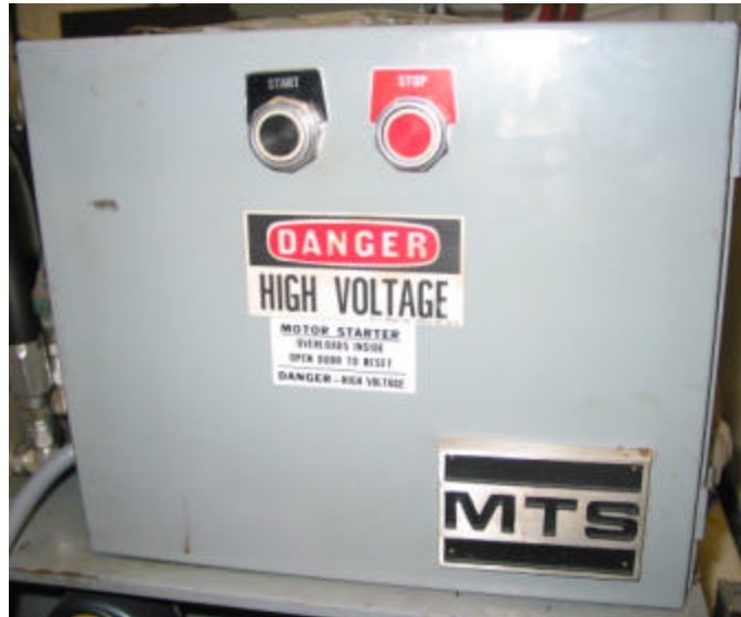
Figure 4 – Hydraulic Power Supply (HPS) Power Panel (located behind and to the left of the load frame).
