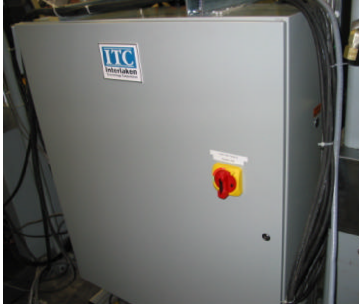
Figure 2 – Main Power Panel 2 (located to the left of the load frame and under Main Power Panel 1).
