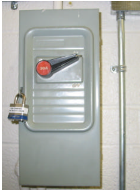
Figure 3 – Main power disconnect switch for pump (located on the wall behind the load frame).
