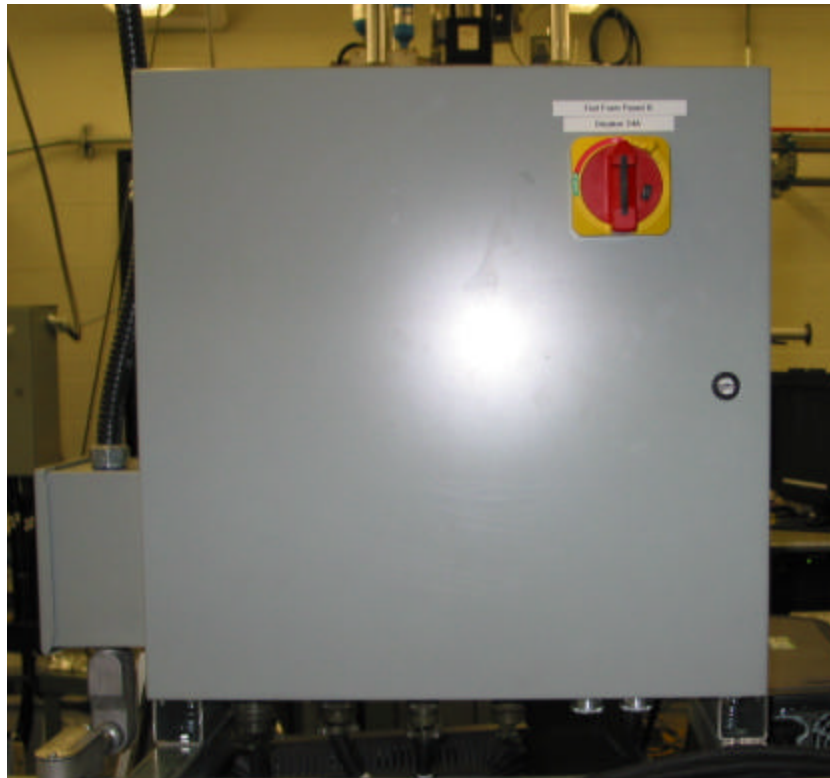
Figure 1 – Main Power Panel 1 (located to the left of the load frame).
